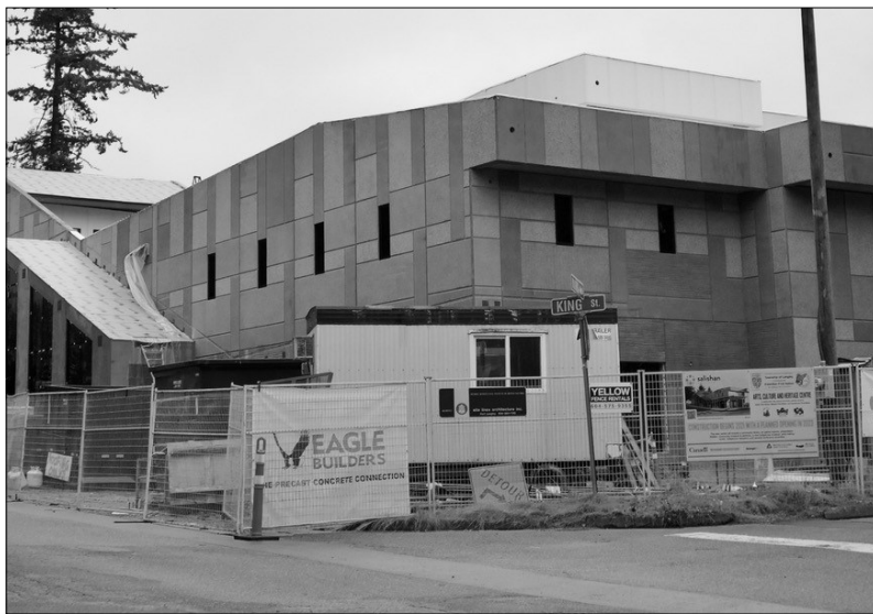
Salishan Place By The River is under construction at the corner of King Street and Mavis Avenue in Fort Langley. Photos: Mark Forsythe.
